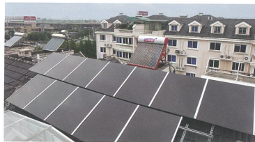
The household solar project on No. 2 Huaxia Road of Pudong New Area in Shanghai (Installed capacity: 1.5 kWp)
