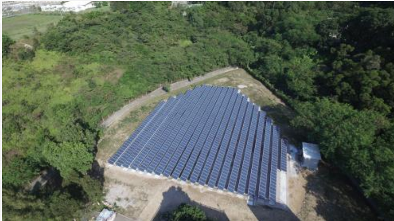
Solar Farm Area C
