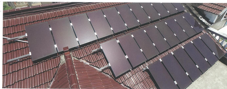
The household solar project in Guoyuan Community of Xucheng Town in Xuyi County of Jiangsu (Installed capacity: 4 kWp)
